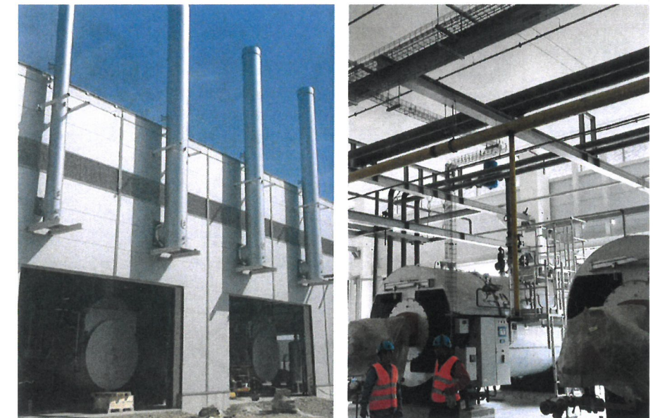
PIPING & EQUIPMENTS MTG PHILIP MORRIS TOBACCO PLANT BOLOGNA - ITALY 2015
