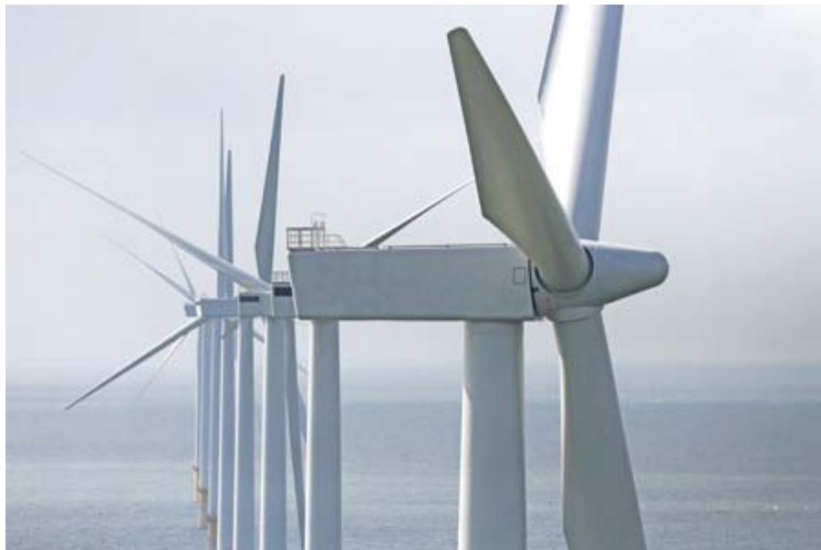
Fig. 14: Offshore 3.6 MW Siemens wind turbines at the Burbo offshore wind site operated by Dong Energy. Source: Siemens.
