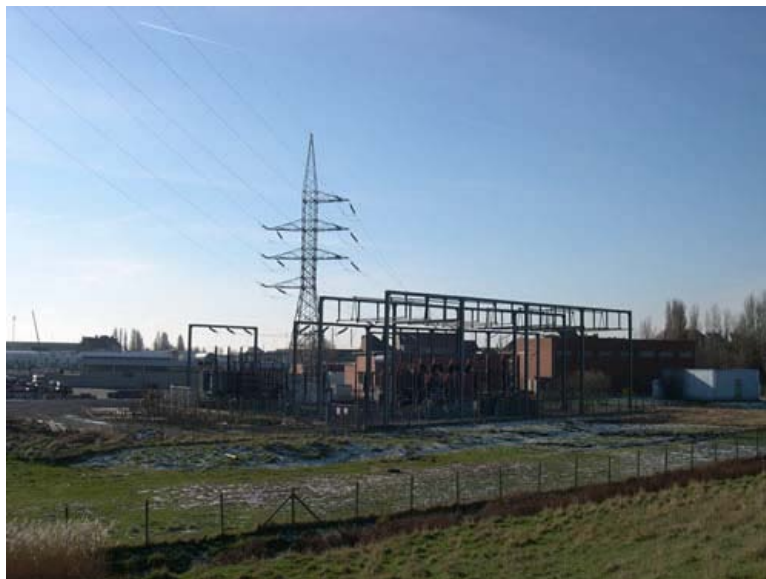
Fig. 51: Onshore switching station for connection to the power grid. Source:
