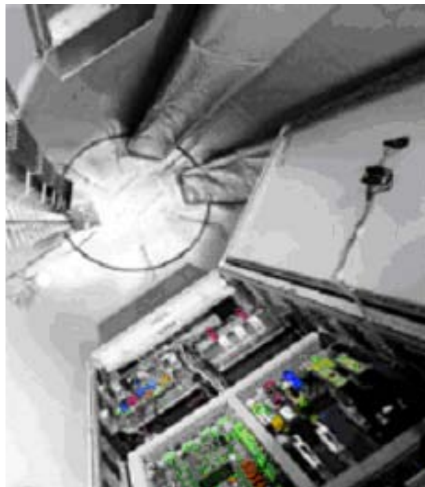
Fig. 28: System controls are located inside the structural tower protecting them from the environmental conditions and from possible intrusion and vandalism.
