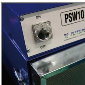
Quadro comandi Electric panel board
