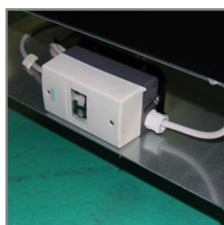
Quadro comandi Electric panel board
