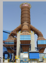
Unisteel Steel Plant Kuwait
